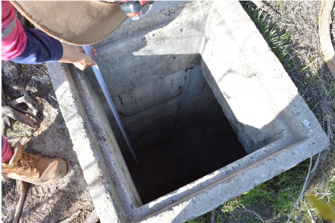
Figure 23: Manhole to water tank, located east of the vehicle track. Scale reaches down 2m. Photo facing east.
