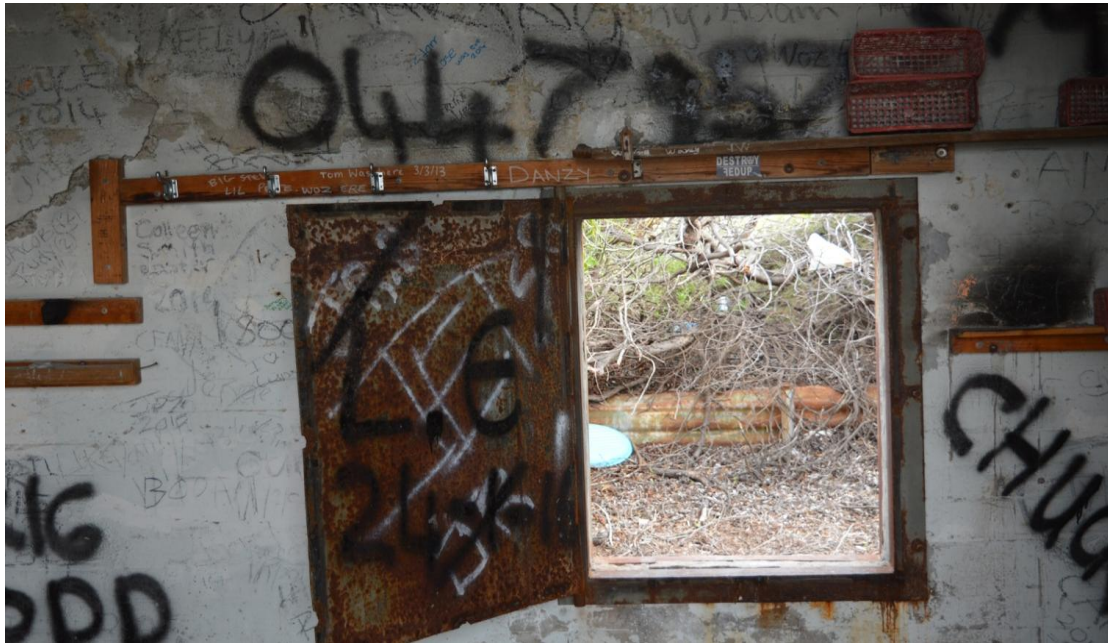
Figure 9: Graffiti on southern interior walls of Igloo B. Photo facing south.
