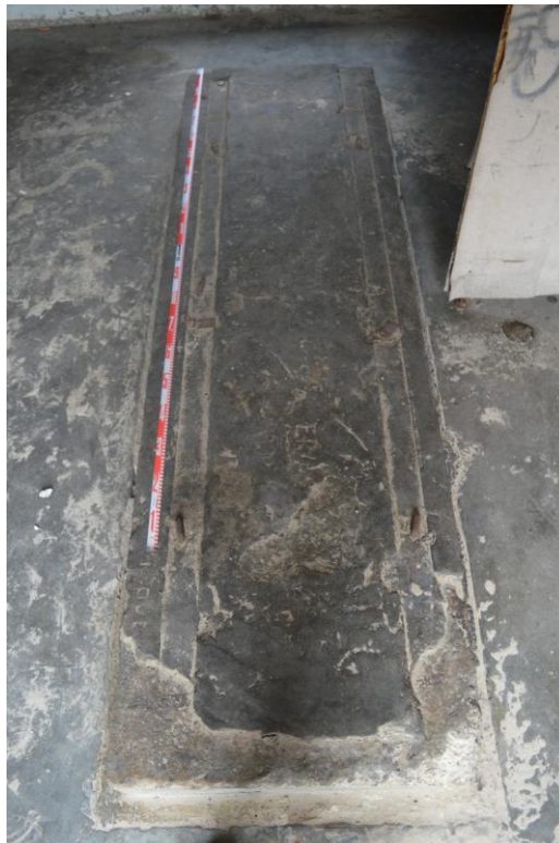
Figure 8: Generator engine bed inside Igloo B. Scale 2m. Photo facing south.
