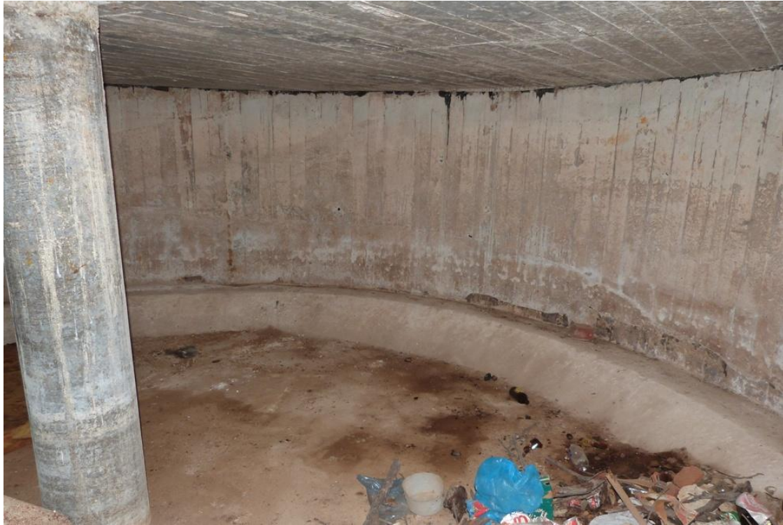
Figure 21: Interior of water tank. Facing northwest. Rubbish has since been collected by volunteers.
