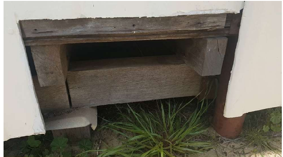
Photograph 14 – Penetrated sections of asbestos outer wall sheeting.
