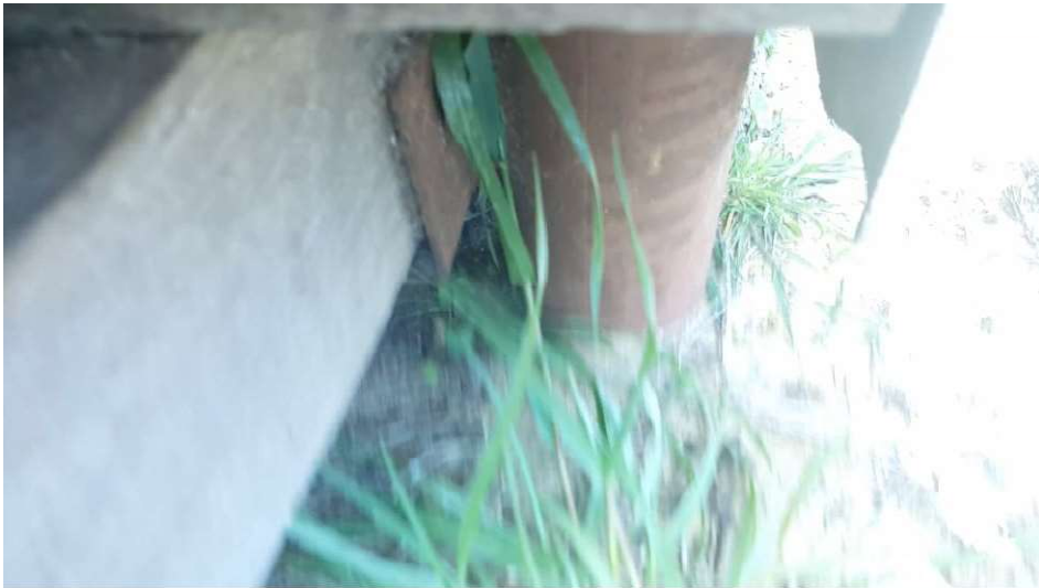
Photograph 13 - Lower sections of the roof supporting columns (Minor Surface rust)
