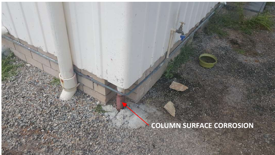
Photograph 5 – Lower sections of the roof supporting columns (Minor Surface corrosion)
