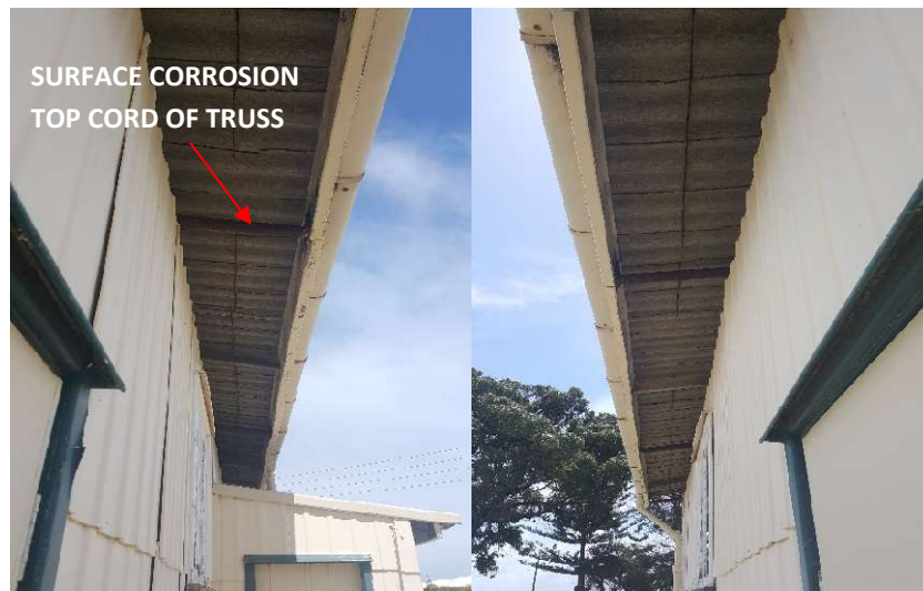
Photograph 11 – Corroded mesh detail within eaves & Surface corrosion to the top cord of the roof truss that supports the timber fascia board
