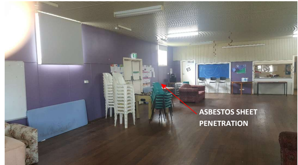
Photograph 16 – Penetrated sections of inner wall sheeting.
