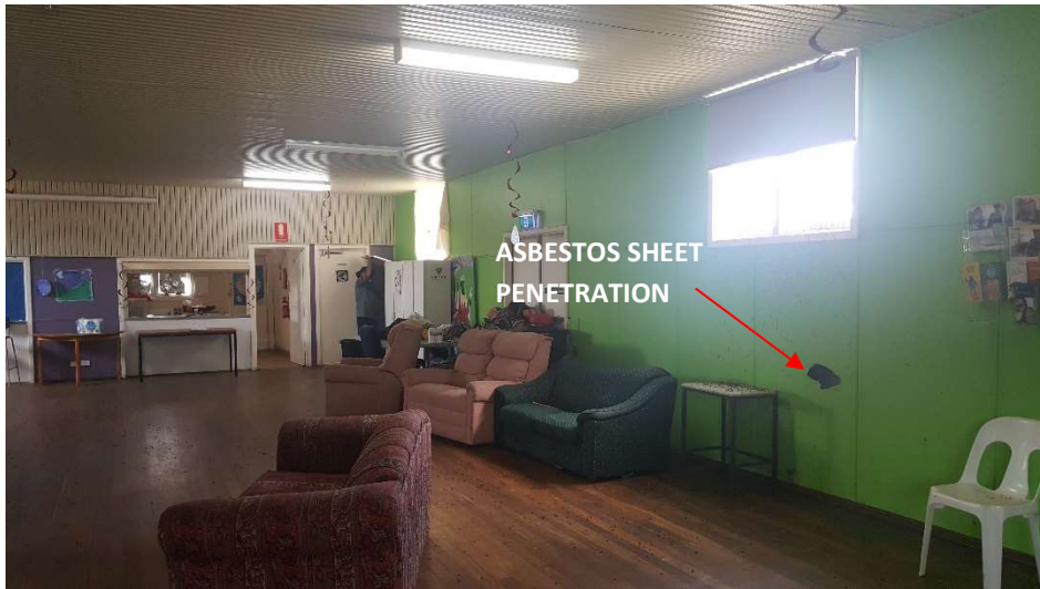
Photograph 15 – Penetrated sections of inner wall sheeting.
