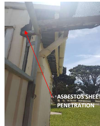
Photograph 12 – Penetrated sections of asbestos outer wall sheeting.
