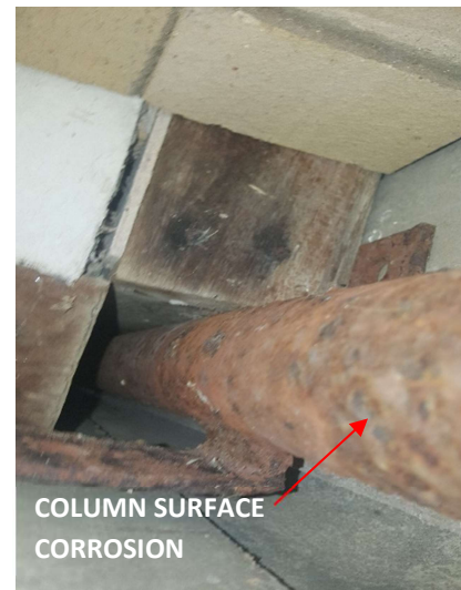
Photograph 6 – Minor surface rust to the lower section of column.
