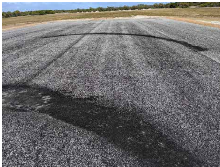
Turing C130 surface damage
