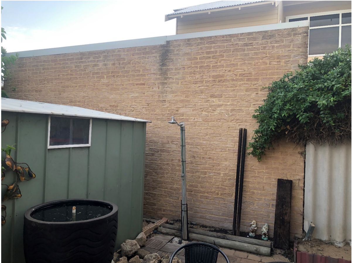
Figure 4: Example of a brick parapet wall against small private courtyard. The parapet wall in this example supports a single car drive-through garage for the adjoining property and is generally more aesthetically pleasing to users of the courtyard than the significantly lower Hardiflex™ default fence.
