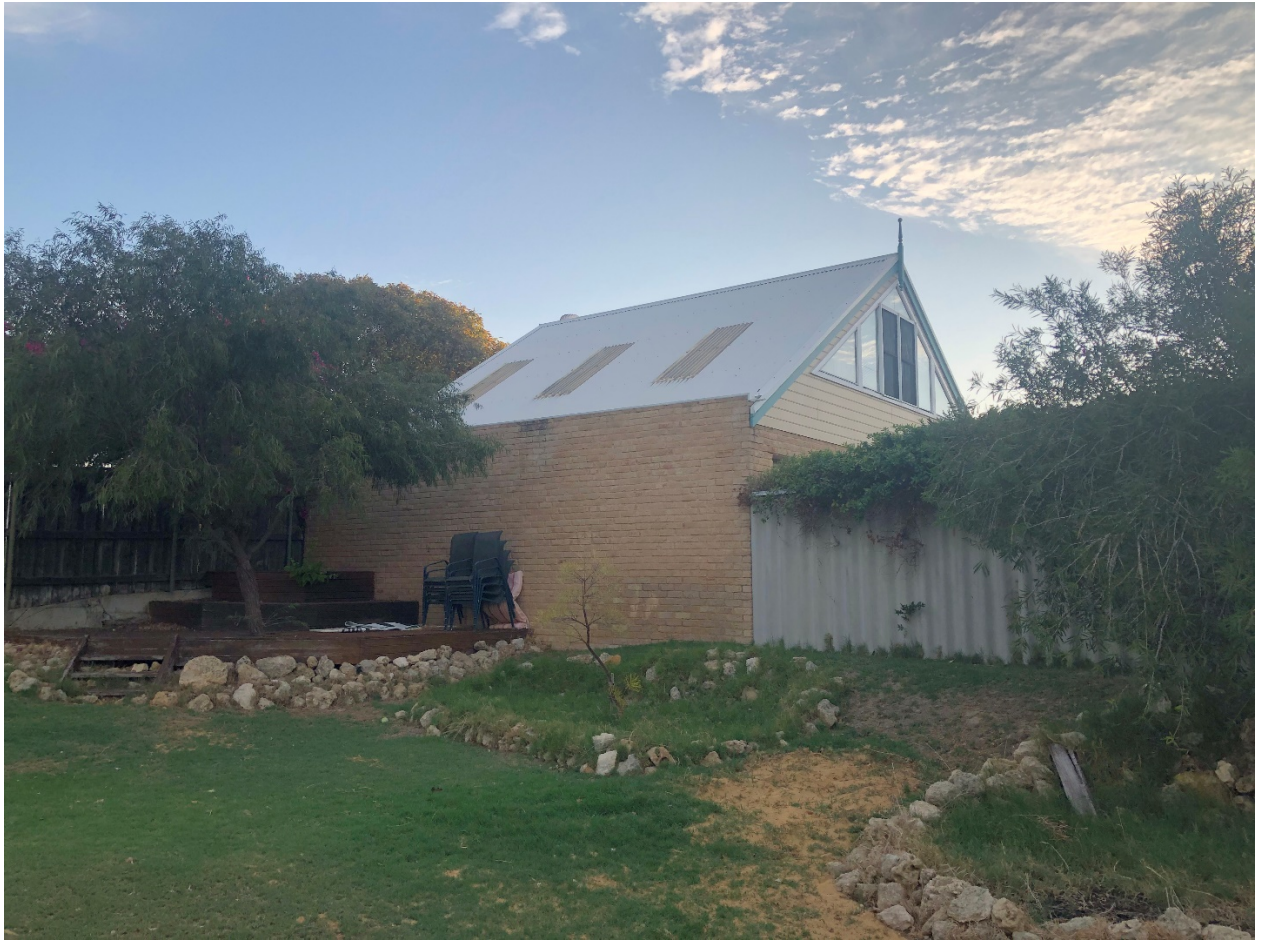
Figure 5: Further example of a parapet wall supporting a more substantial structure (2/3 car garage and loft accommodation). Once again, the parapet wall forms a generally aesthetically pleasing boundary solution enabling the adjoining property to develop the structure they wish to.
