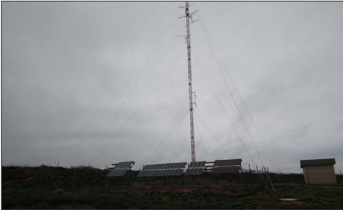
Figure 1 Guyed mast example with solar array at Bullara (Exmouth)
